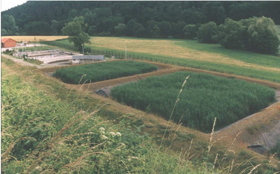
Reed bed dewatering in Naumburg, beds 1 and 2, activated sludge treatment plant in the background
